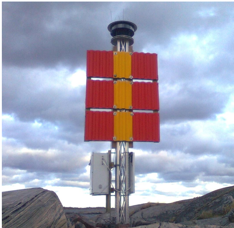
Picture 6. Sector Lantern E8262.RWG-LB-F6337 installed at Ronnbackskär, Finland.
